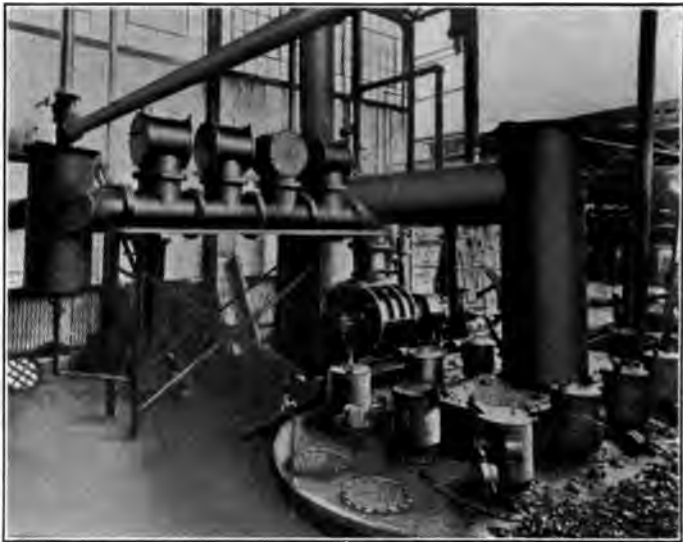
FIG. 232.—Charging floor Smith producer showing tar extractor.
